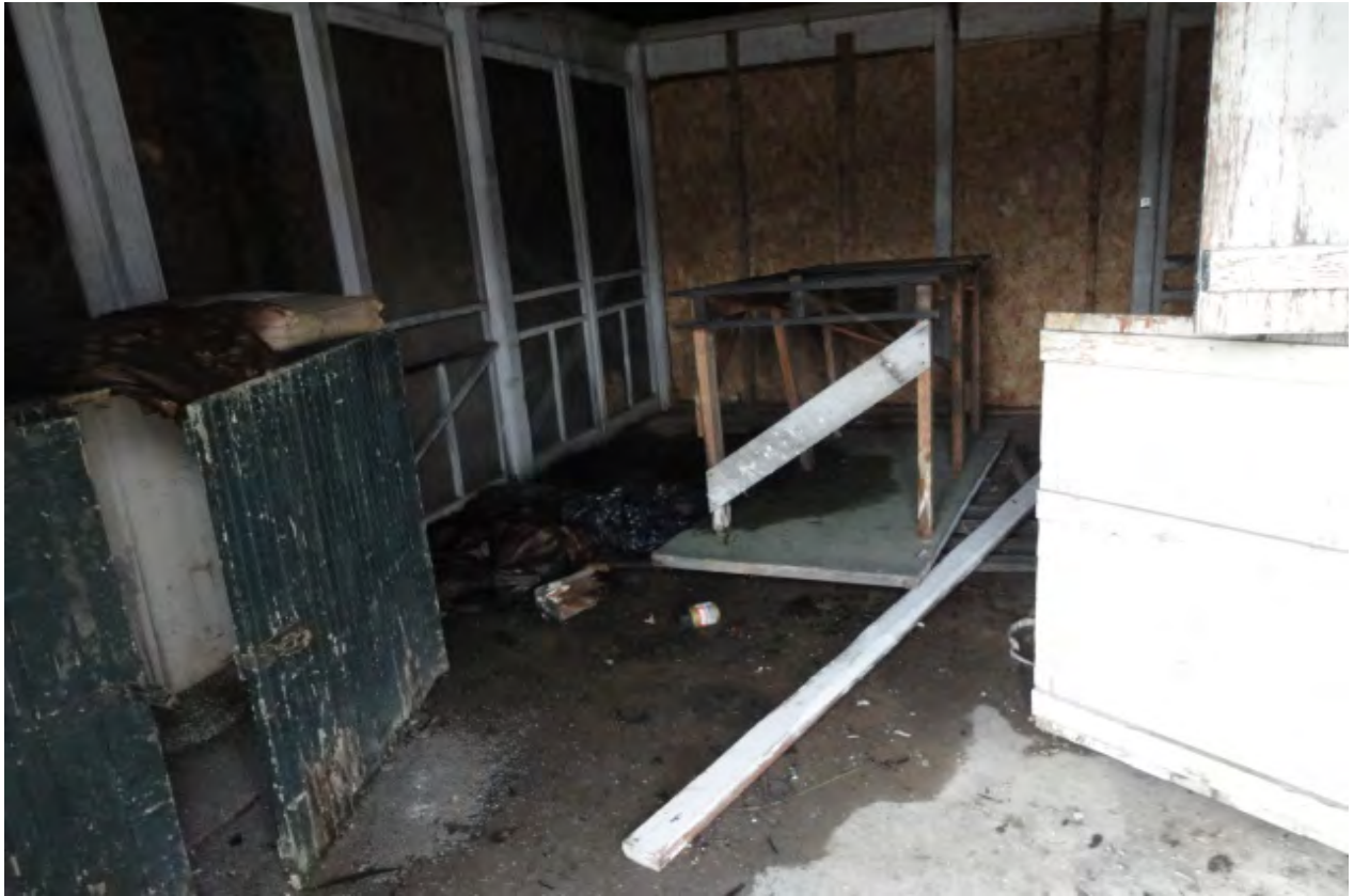
Photograph 21: View of the interior of the small unit storage building near the Site's northwest corner.
