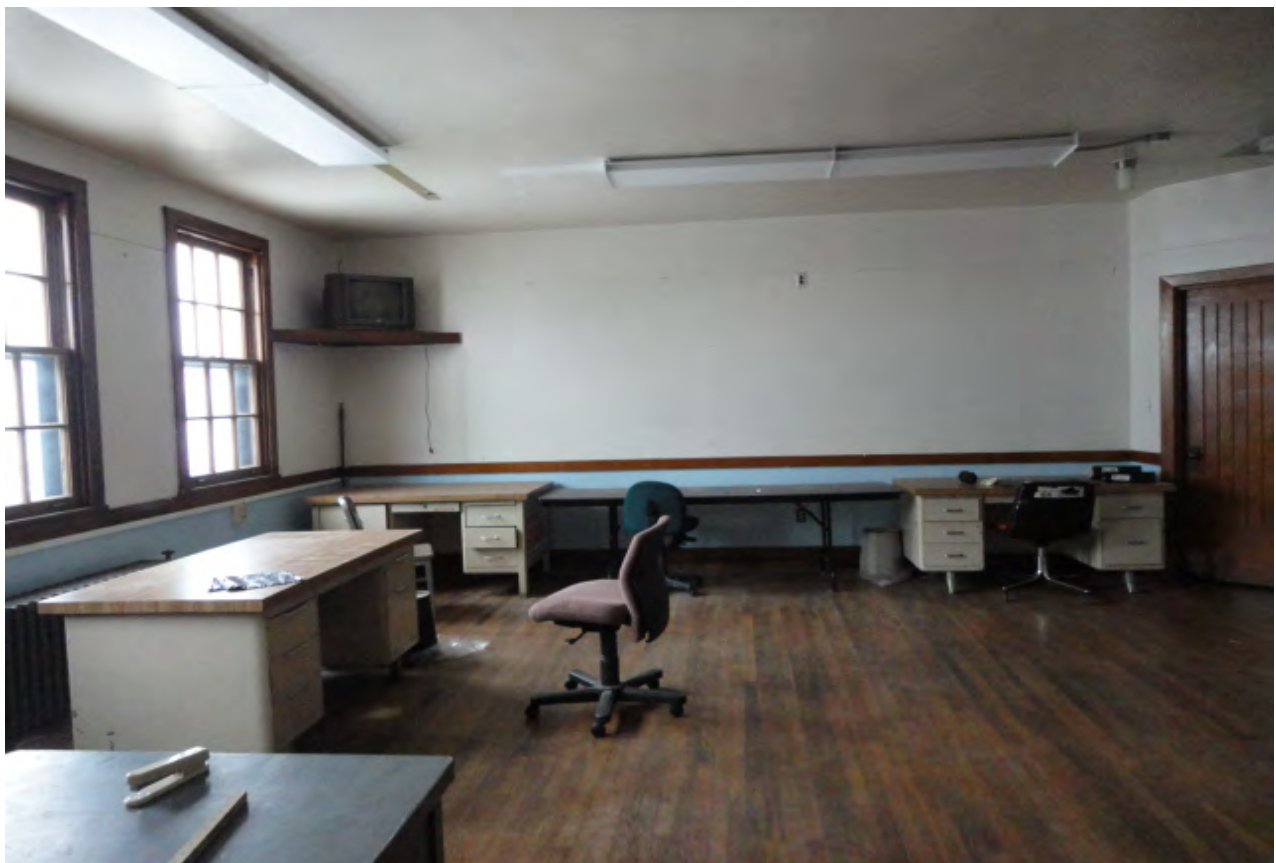
Photograph 14: View of the large 2 nd floor office space. Note the television set remaining on the east wall.
