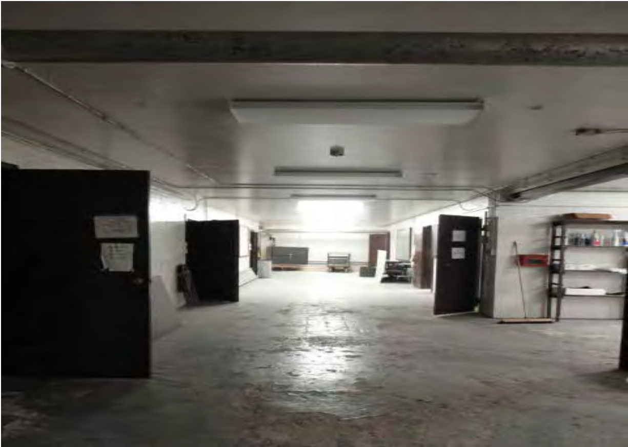
Photograph 7: View to the north of the former IFR in the RC basement.
