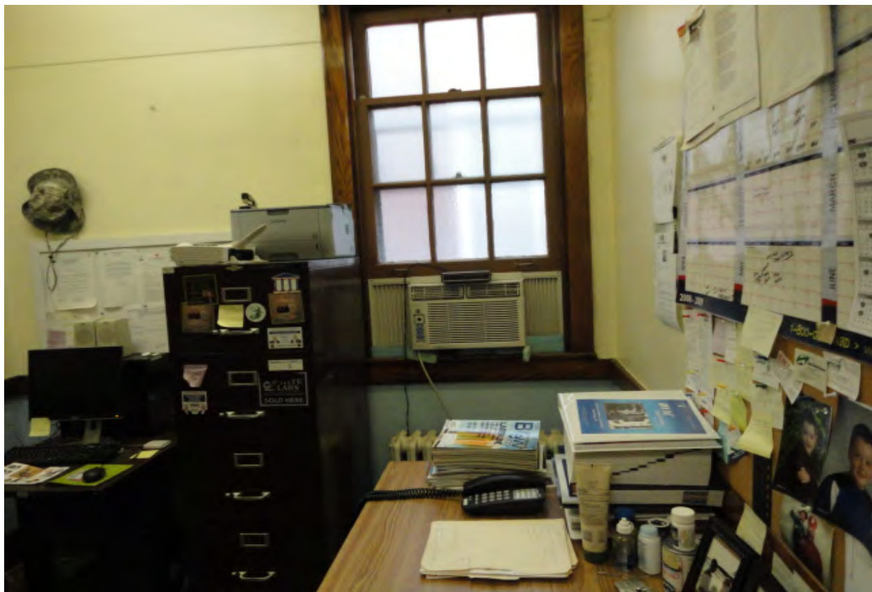
Photograph 18: View of remaining window-mounted air conditioning unit in the second floor maintenance office.
