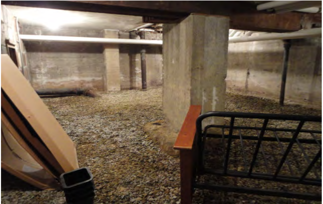
Photograph 11: View of storage crawlspace in the northern side of the basement where ACMs were previously abated.
