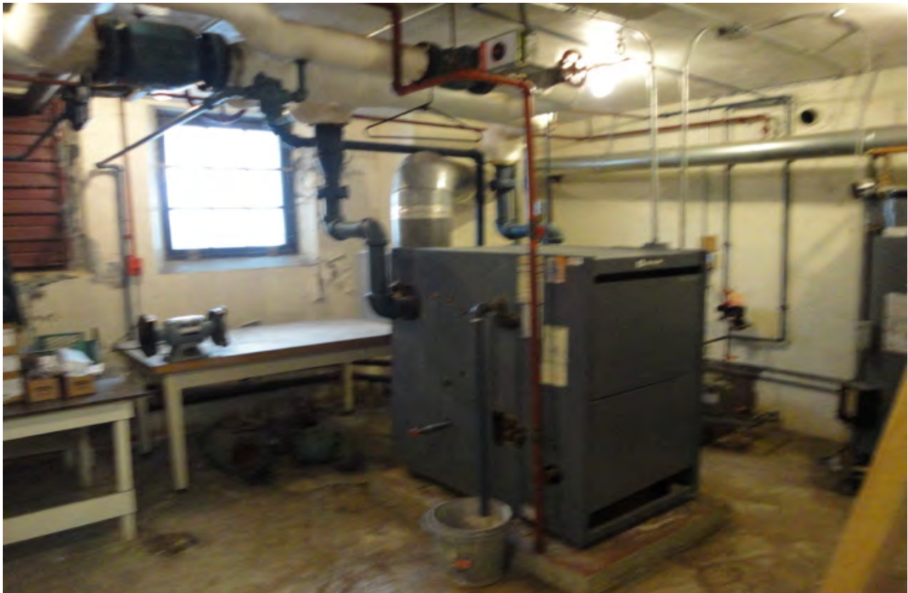
Photograph 6: View of the boiler room in the RC basement.
