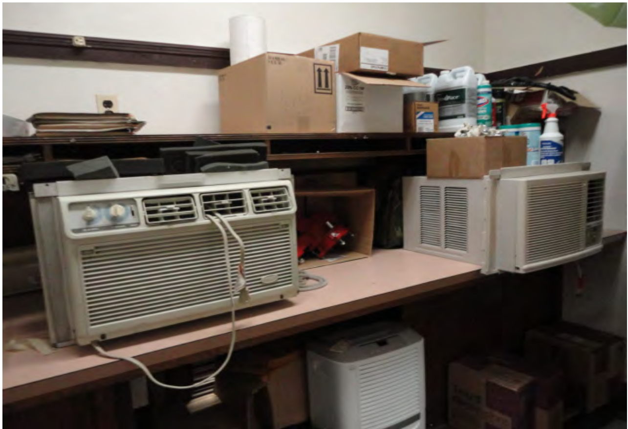
Photograph 13: View of window-mount air condition units in a first floor maintenance storage room.
