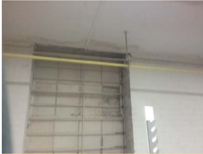
1. Water damage on ceiling in the Gym
