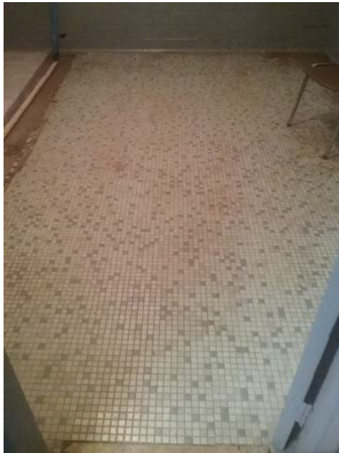
2. Damaged potential asbestos containing floor tiles
