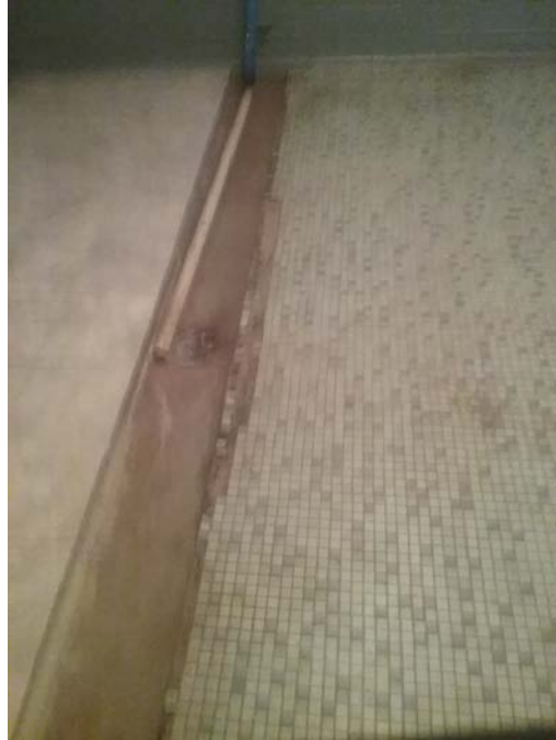
3. Damaged potential asbestos containing floor tiles
