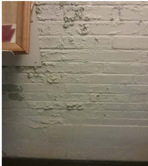
4. Suspect water damage on wall in hallway near main entrance
